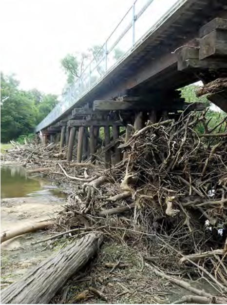
Bike trail bridge debris
