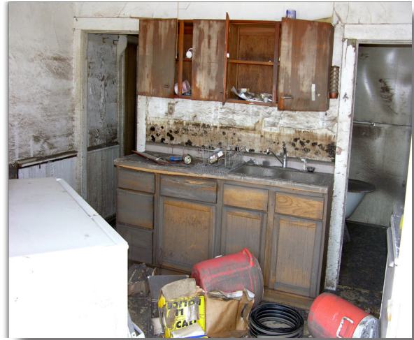
Figure 5-1. A Cedar Rapids home damaged by the 2008 flood. Residents returning to muck out and gut their homes after such events are faced with extensive mold growth, chemical and microbial pollutants, and other potential health hazards. With current rises in precipitation and streamflow, floodplain residents may be increasingly exposed to such hazards. (Photo credit: Linn County Public Health Dept.)
