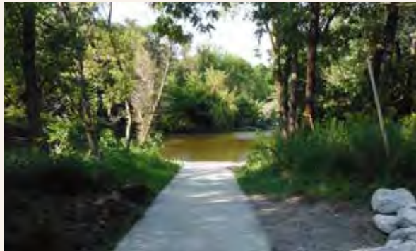
Figure 24 This existing launch is upstream of the dam and has been damaged at the river edge by high flows.
