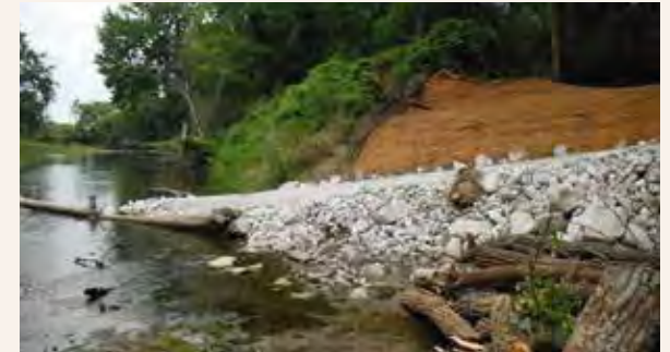
Figure 21 A portage trail around this dam was constructed by Iowa Conservation Corps volunteers in 2014.
