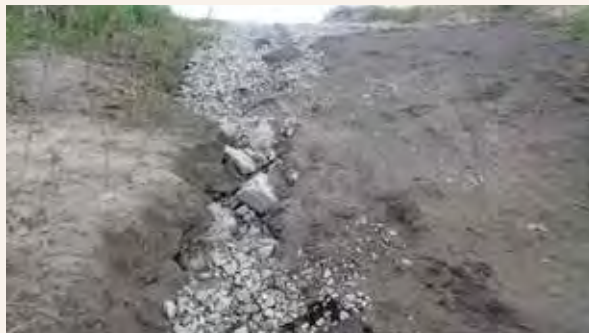
Figure 28 This view of the CJ Shrek launch from the river illustrates the erosion caused by drainage from the access parking area. The proposed replacement launch is concrete and includes resolution of stormwater drainage patterns.
