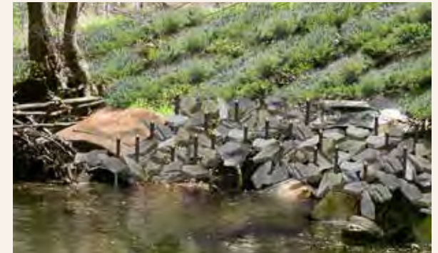
C3.A Following removal of surface material, rip rap should be carefully placed below the bankfull elevation in the gaps where the streambank is newly exposed. Revegetation can then occur.
