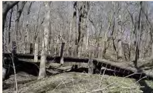
R3.F This bridge was established and has been repaired multiple times with volunteers. Replacement with a more formal bridge is recommended.
