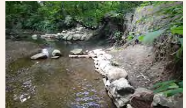
C2.C J-Hook rock structures are minimally-invasive structures keyed into the streambank. The rock formation redirects the thalweg (the deepest part of the channel) away from the eroding streambank.
